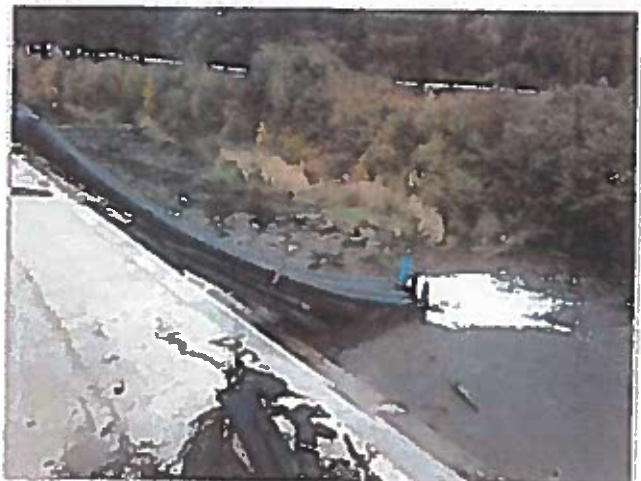
FIGURE 9 - OUTLET OF SIPHON WITH VALVES
