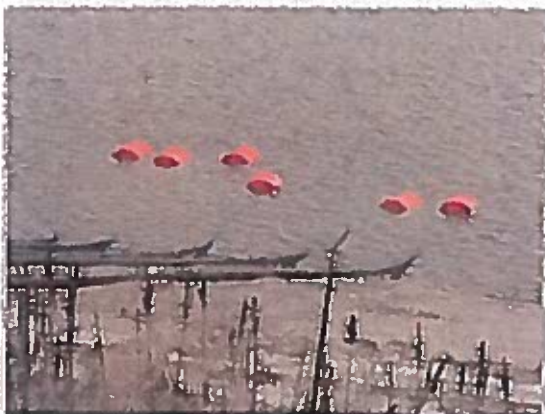
FIGURE 22 - SUBMERSIBLE PUMPS AND FLOATATION
