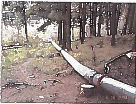
FIGURE 12 - CRUSHED ALUMINUM PIPE
