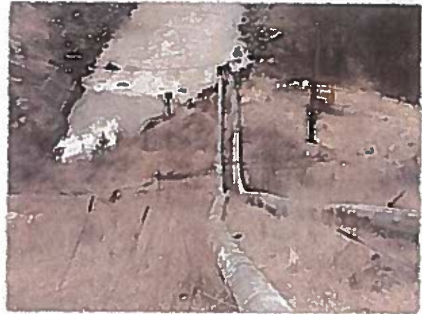
FIGURE 21 - DISCHARGE PIPE RUNNING DOWN CROW DAM EMBANKMENT
