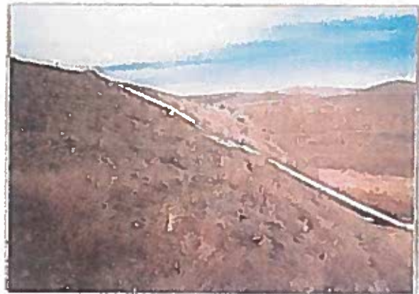
FIGURE 26 - COLLAPSED PVC PIPE
