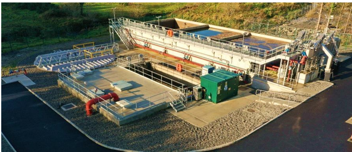
Figure 10: Killala waste water treatment plant
