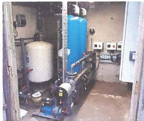
FIGURE 4: Upgraded treatment system at Coole Group Water Scheme, County Galway
