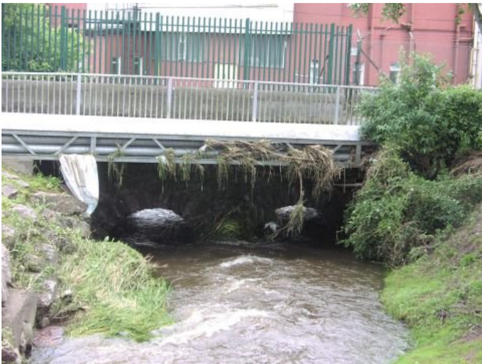
Photo showing small two arched bridge downstream of large culvert in previous photo. Note debris gathered on pipes. Based on the Lee CFRAMS Channel & Cross Section Survey (7BRI_1425), the flood level indicated by this debris would be about 18.1m to 18.2m OD Malin, but this would be a rough estimate and would need to be surveyed before being relied on.
