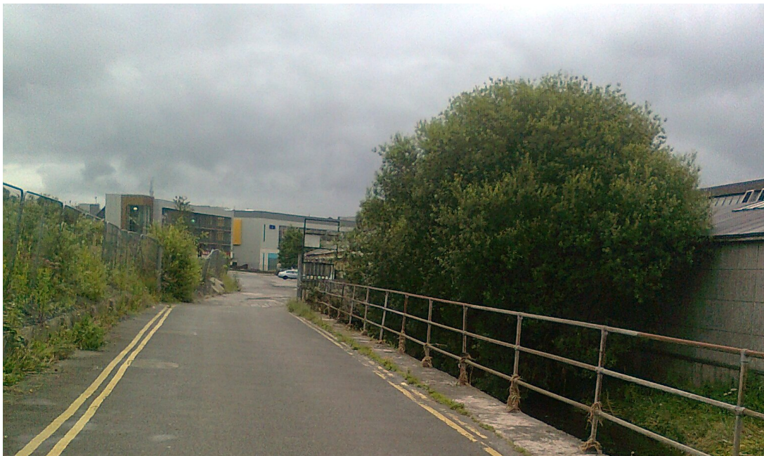
Photo looking downstream toward entrance to Culvert at Rear of Millfield Industrial Estate. Lee CFRAMS channel cross section 7BRI_991 is just upstream of the culvert entrance beyond the trees in the photo. Estimated level of flood here about 15.7m OD Malin. Again, this to be taken as a rough estimate only.
