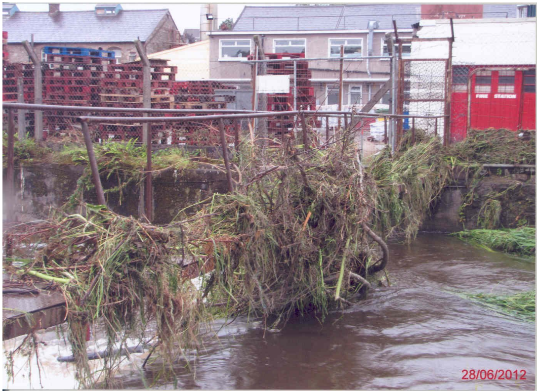
Photo Given to me by member of the Public. Based on the Debris level in this photo & the Lee CFRAMS Channel & Cross Section Survey (7BRI_1072), the flood level upstream of this footbridge would have been about 15.6m OD Malin. This should be regarded as a rough estimate, needing to be confirmed by survey, as the whole structure is not recorded in the Survey.
