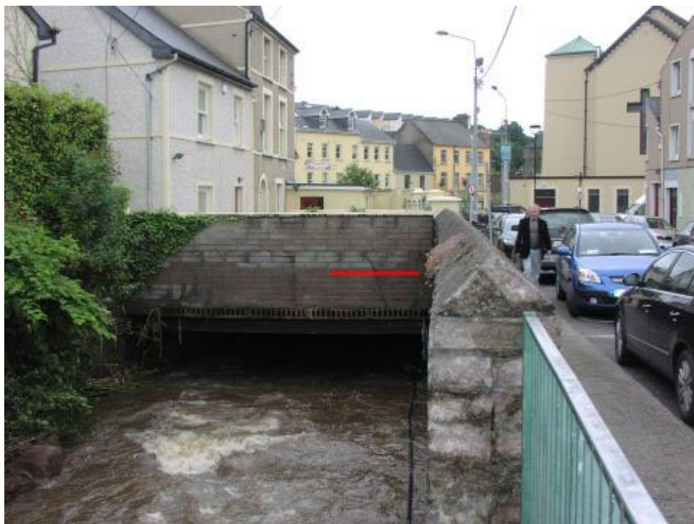
View of entrance to Orchard Court culvert after flood level reduced. Red line indicates level described as observed earlier. Based on Lee CFRAMS (7BRI_93) survey drawing this approximates to a level of about 9.4m OD Malin, and it is about 1.1m higher than the soffit level of the culvert entrance.
