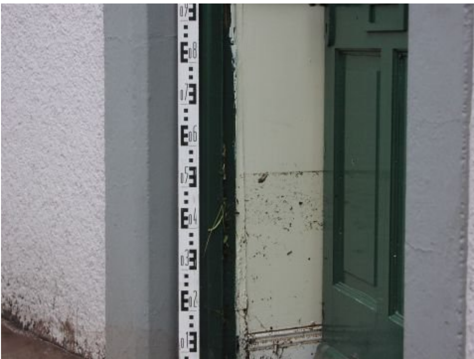
View showing depth of flooding in a house in Thomas Davis Street, (just over 0.5m).
