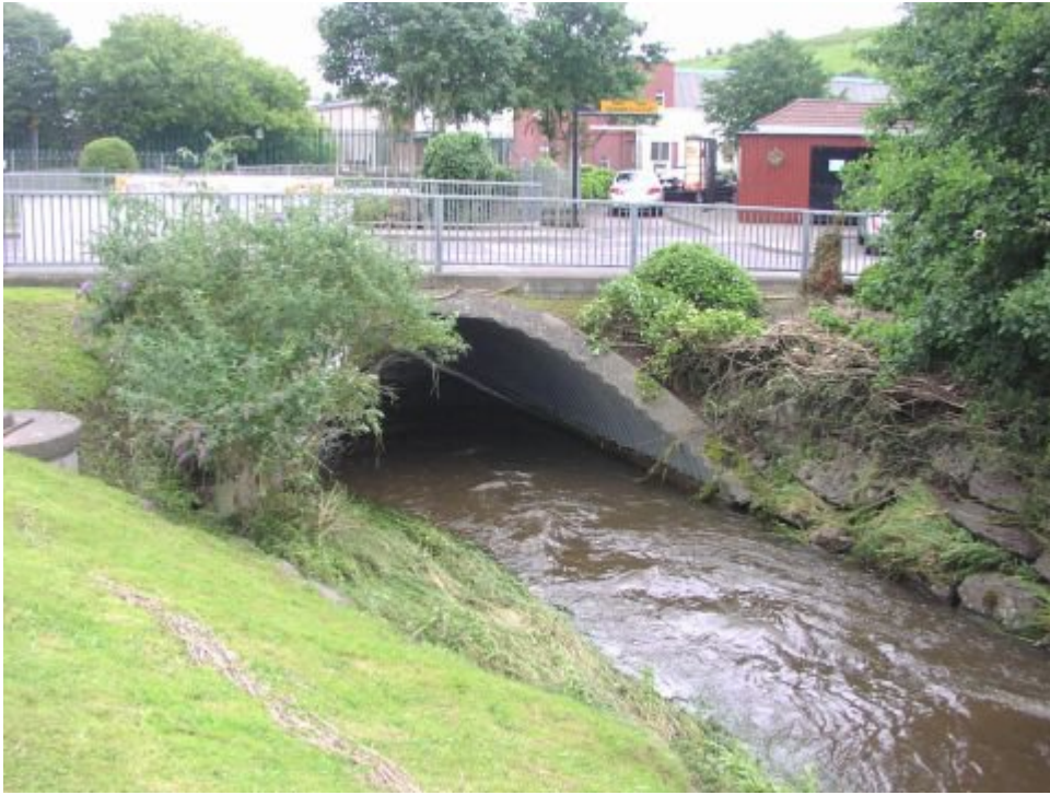
Large culvert on River Bride to east of Topaz filling station and Mc Donalds. Note tide line in left foreground and debris gathered on right bank.
