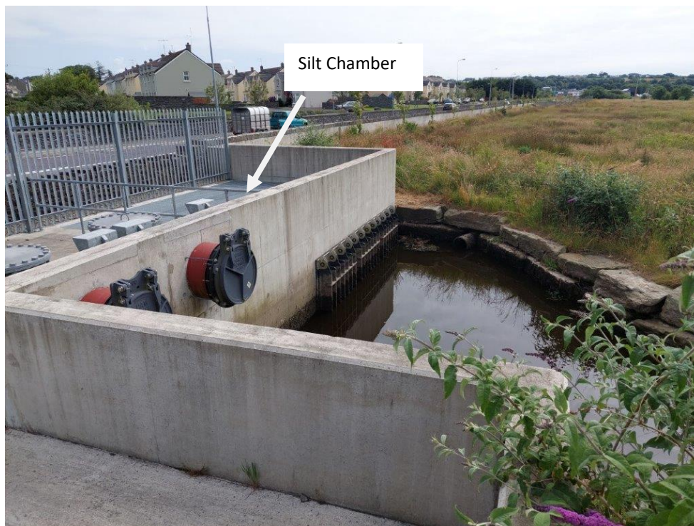
Photo: Schull Road PS Silt Chamber
