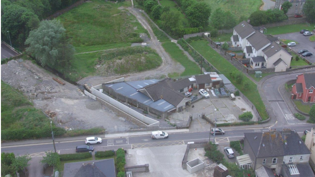
Photo: Townsend Street U-Channel & Culvert (construction photo). Chamber access visible just inside Drainagh Co-op gate
