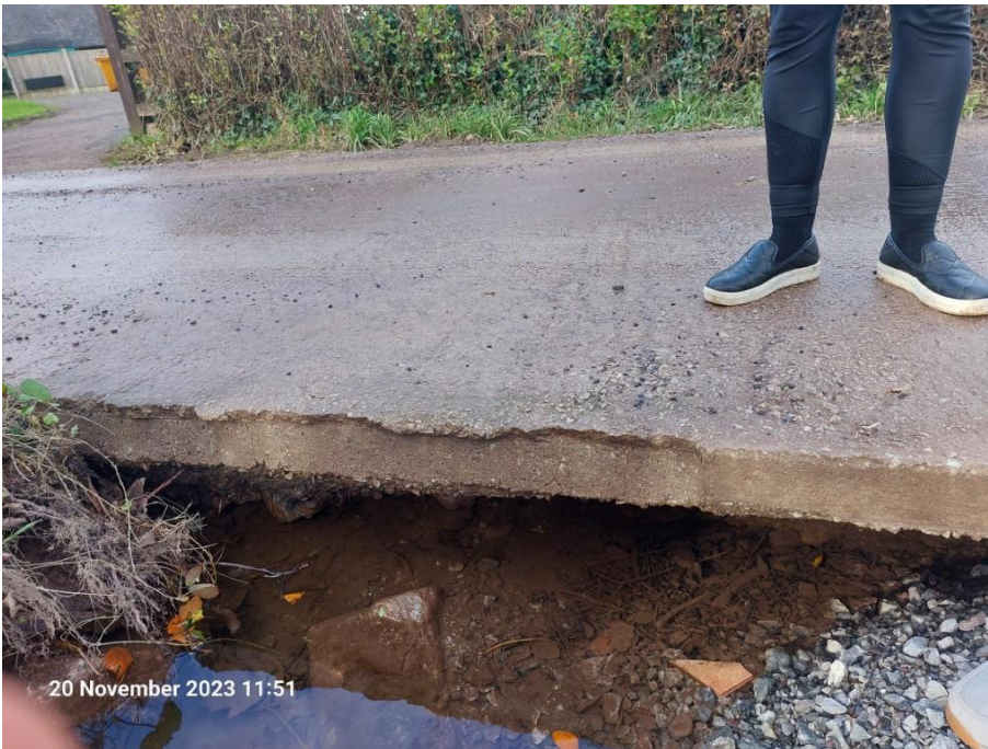
Figure 22: Broomfield Ridge undermined
