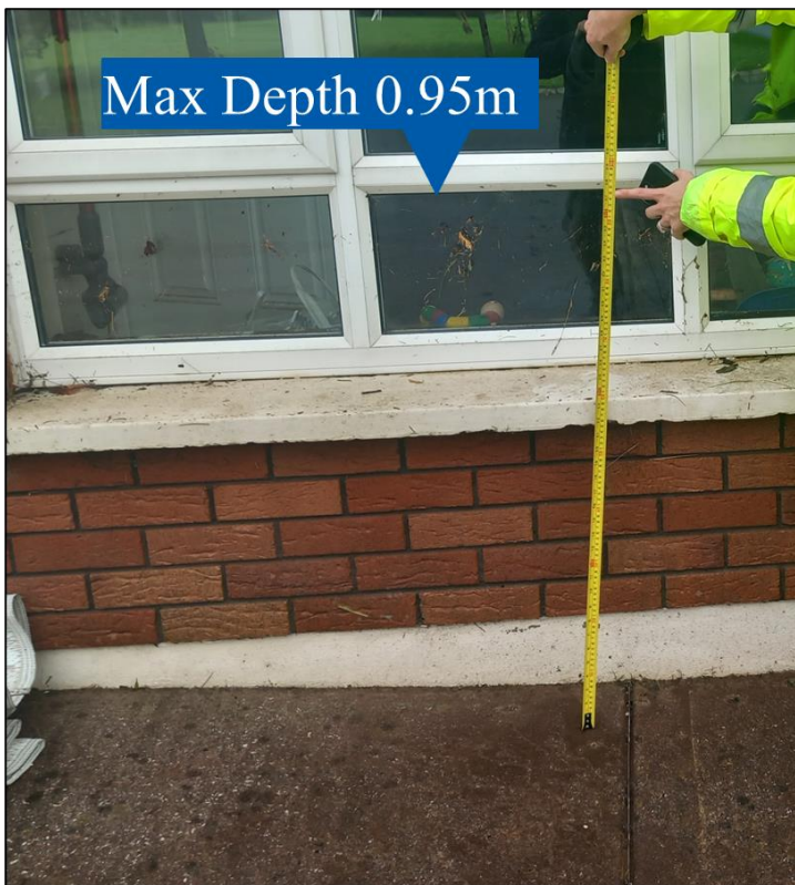
Figure 15: Wrack Mark at No. 13 Riverwalk
