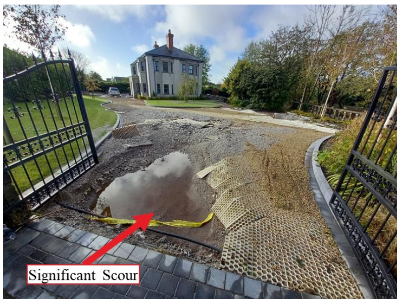
Figure 24: Significant Scour: Entrance to Property Immediately downstream of Moore's Bridge (left bank)
