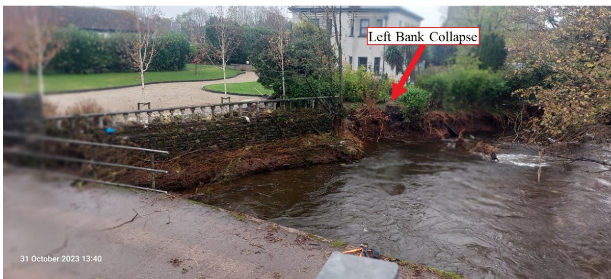
Figure 21: Collapsed Left Bank Downstream of Moore's Bridge
