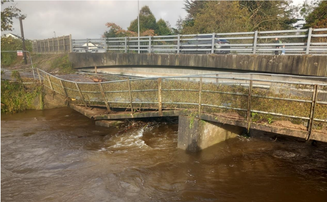
Figure 18: Moore’s Bridge Collapse- Image taken post Storm Babet (19/10/2023)
