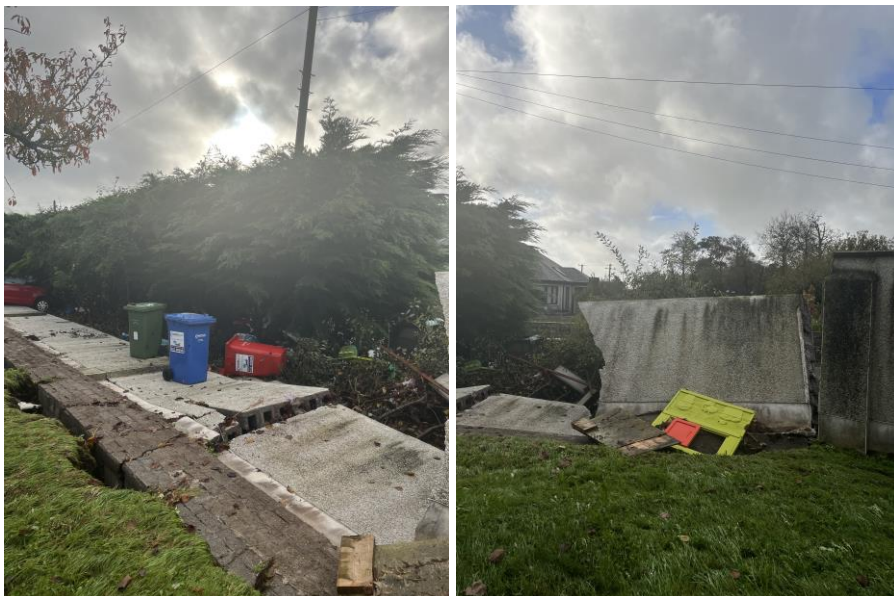
Figure 10: Wall failure at rear of First Steps Creche
