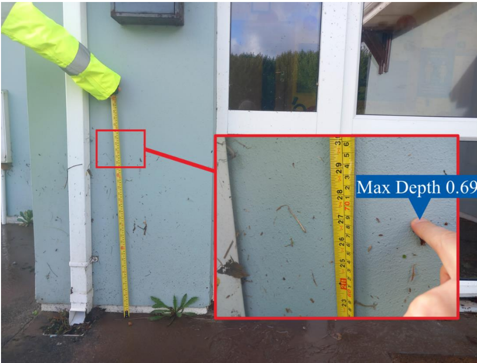
Figure 12: Wrack Mark at entrance to First Steps Creche
