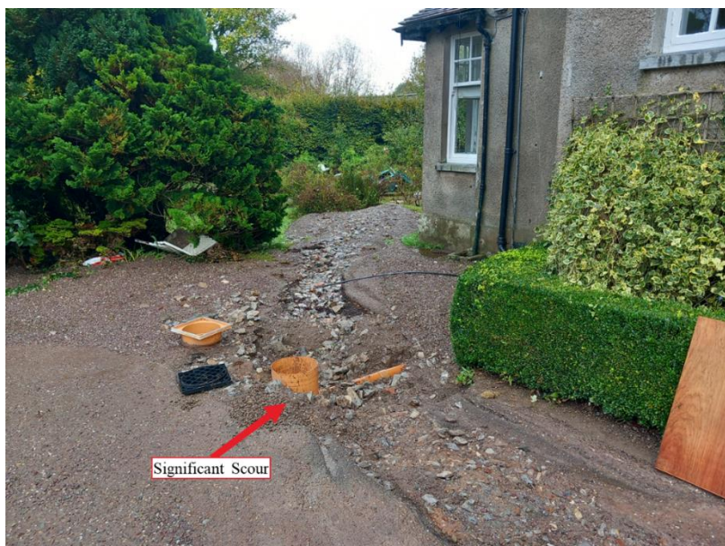
Figure 25: Significant Scour: Property downstream of Moore's Bridge (Left Bank)- Southeast corner of property
