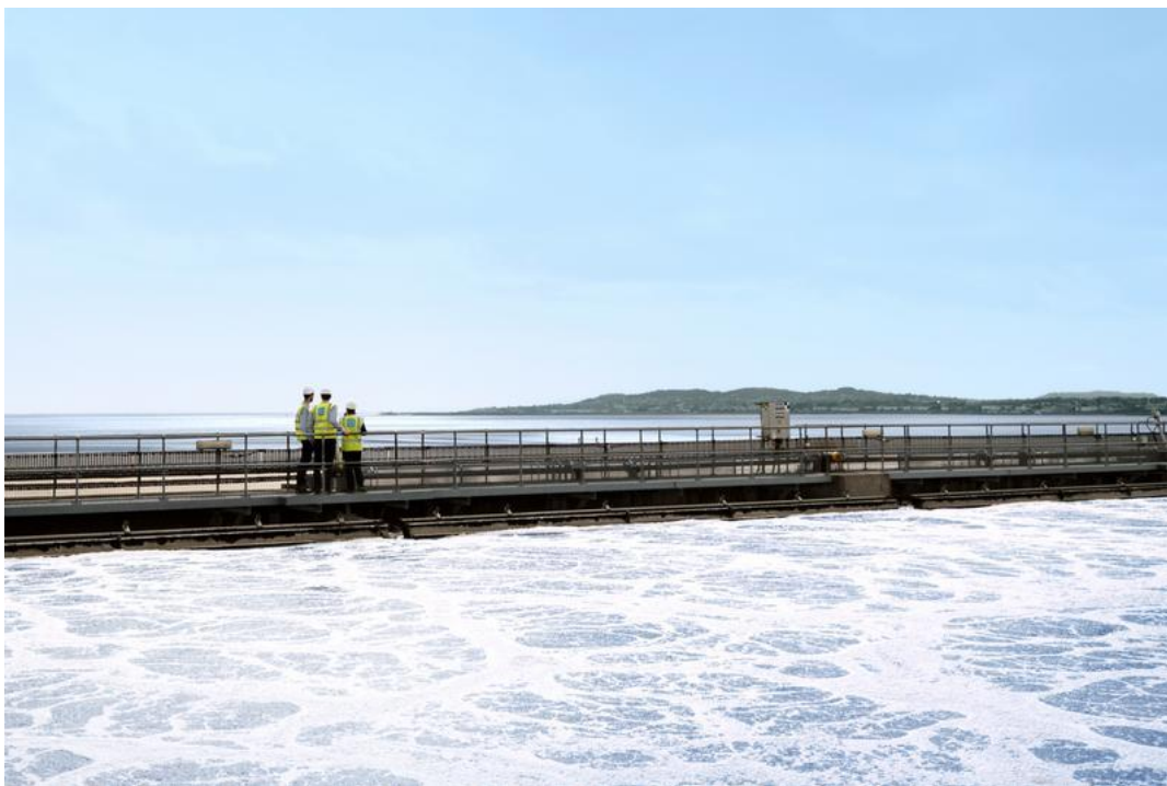
Shanbally WWTP, Cork Lower Harbour
