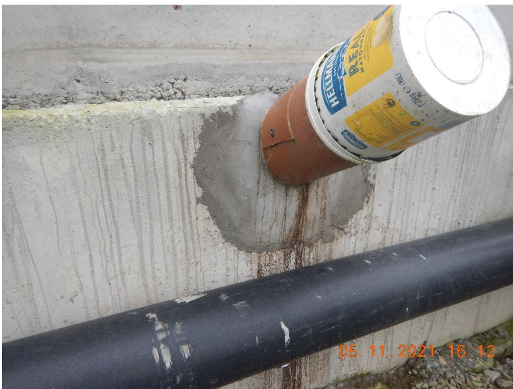
Photo 8; External wall of pig house.
