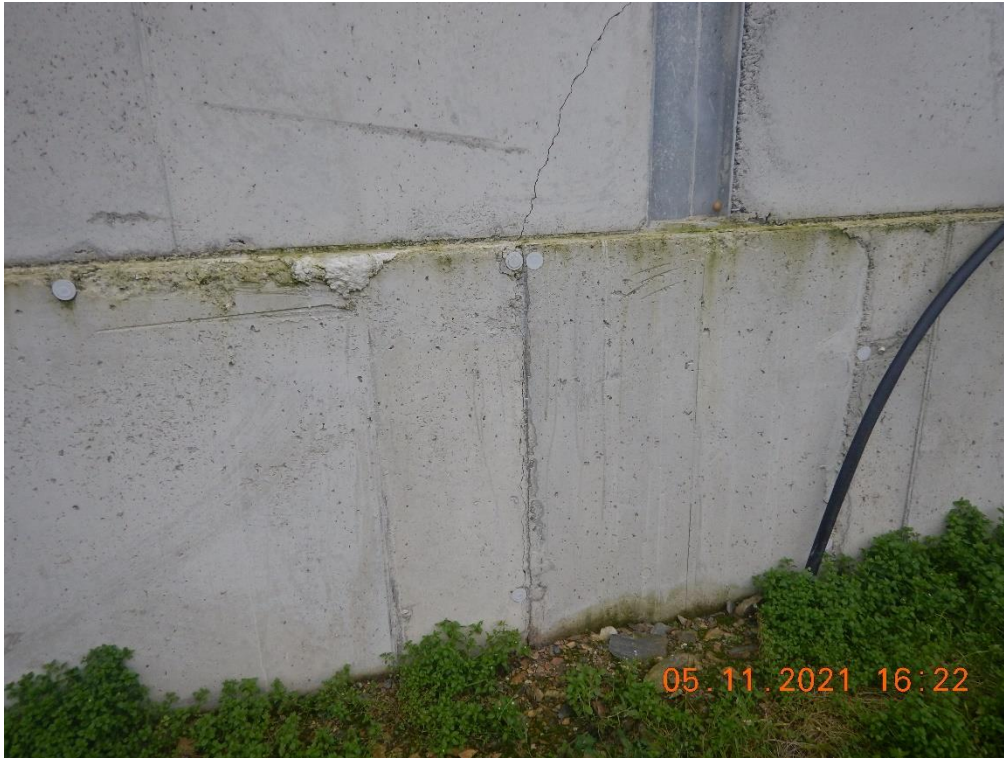
Photo 5; External wall of pig house.
