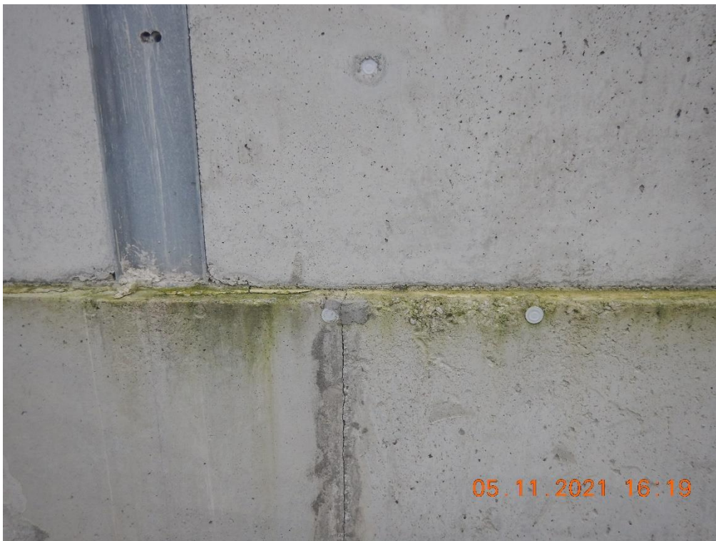
Photo 2; External wall of pig house.
