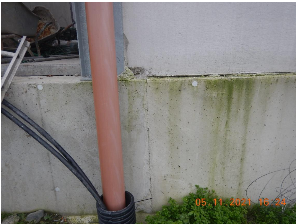
Photo 6; External wall of pig house.
