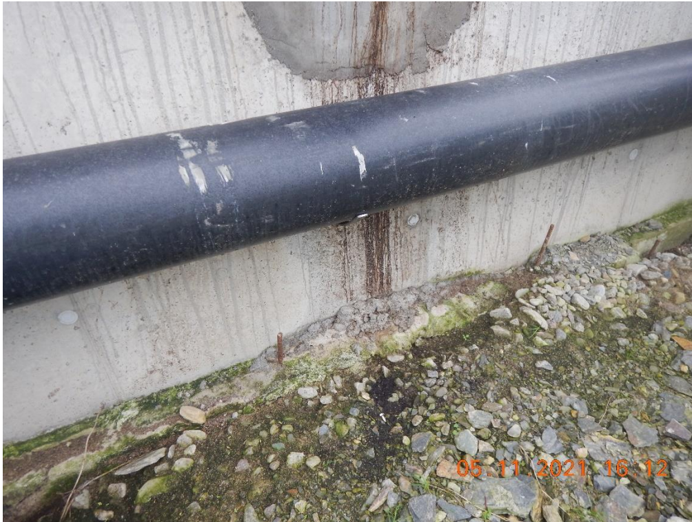
Photo 9; External wall of pig house.
