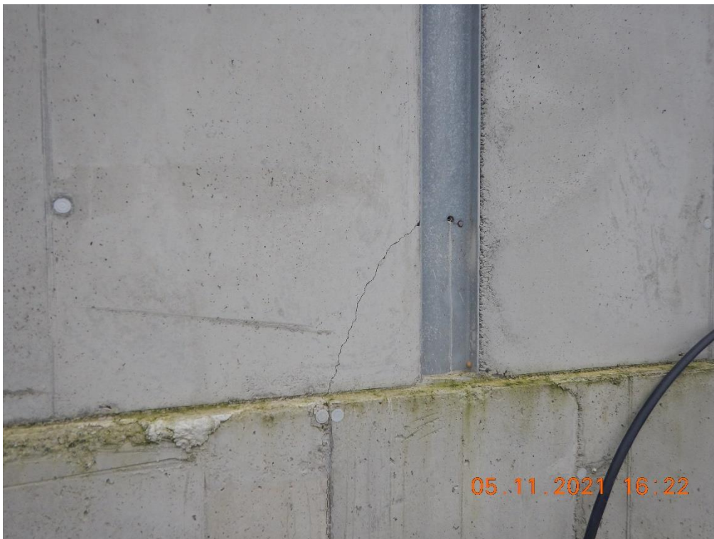
Photo 4; External wall of pig house.
