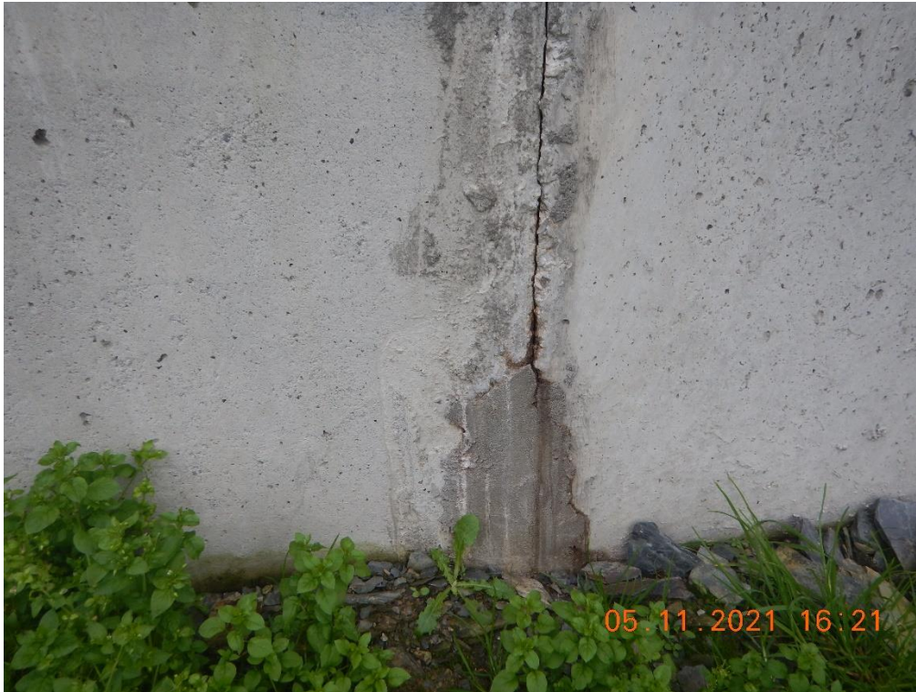
Photo 3; External wall of pig house.
