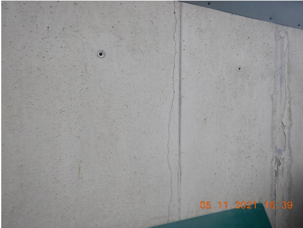
Photo 7; External wall of pig house.
