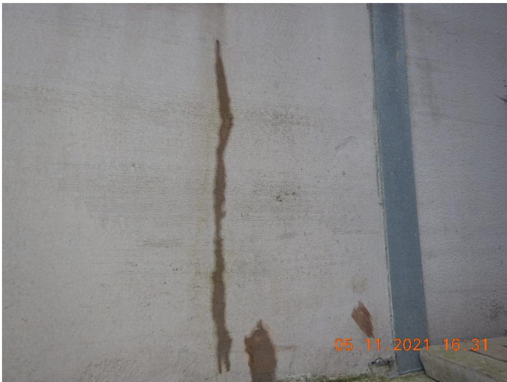
Photo 10; External wall of pig house.
