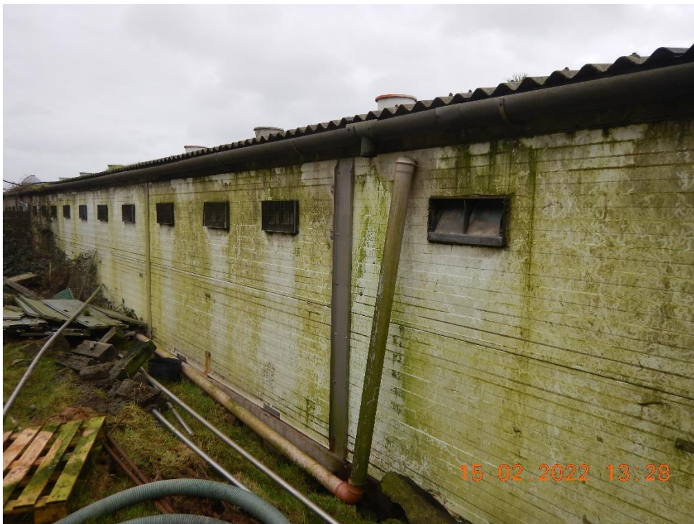
Photo 6; Photograph of disconnected downfall pipe on site.
