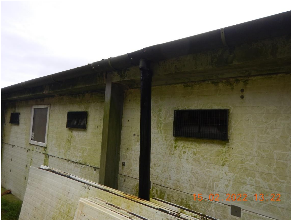
Photo 5; Photograph of disconnected downfall pipe on site.
