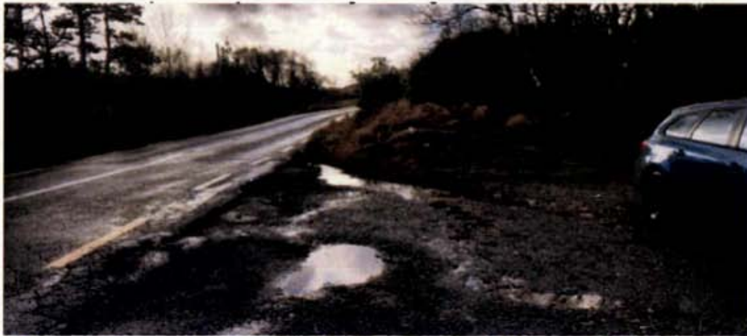
Plate 2: Derryclare forestry access - looking south along R344 (Source: Alan Lipscombe FI Response - Plate 2)
