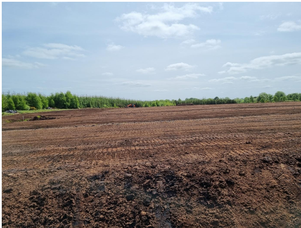
Photo 4: Recently cleared area at southern section of peatland, with excavator noted in the distance.
