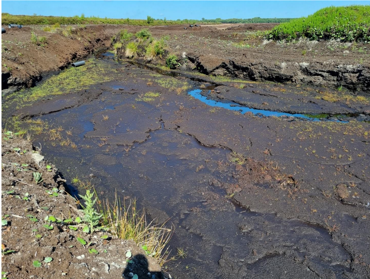
Photo 6: Significant accumulation of solids noted in drainage network at the peatland.
