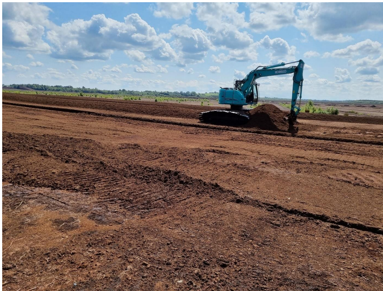
Photo 9: Photograph showing excavator and rows of 'ridged' milled peat on the peatland.
