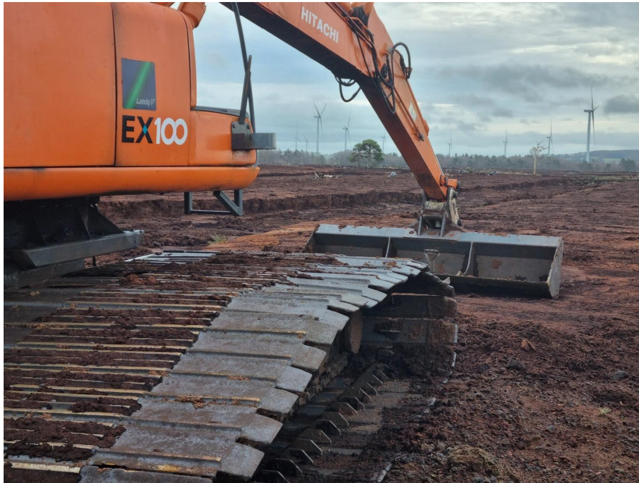
Photo 3: Excavator parked on the western/north western section of the peatland where clearing, drainage and preparatory works had recently taken place.
