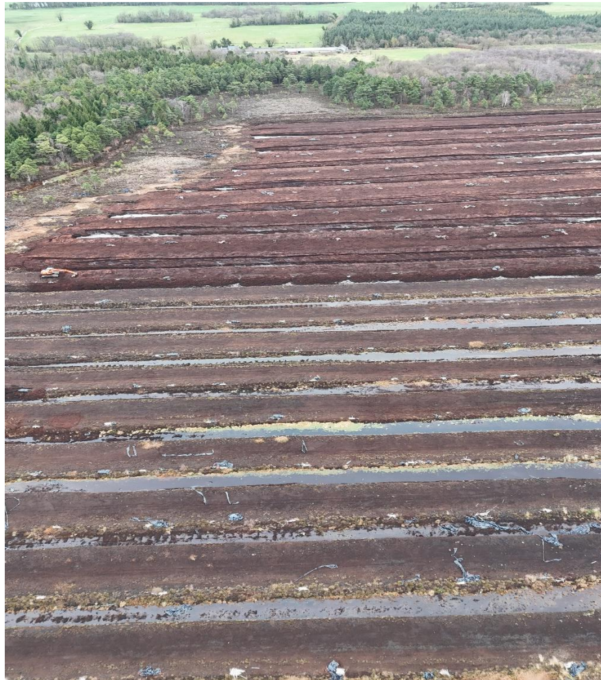
Photo 2: Aerial photograph showing the western/north western part of the peatland where clearing, drainage and preparatory works had recently taken place (note excavator parked on extreme left of photo).
