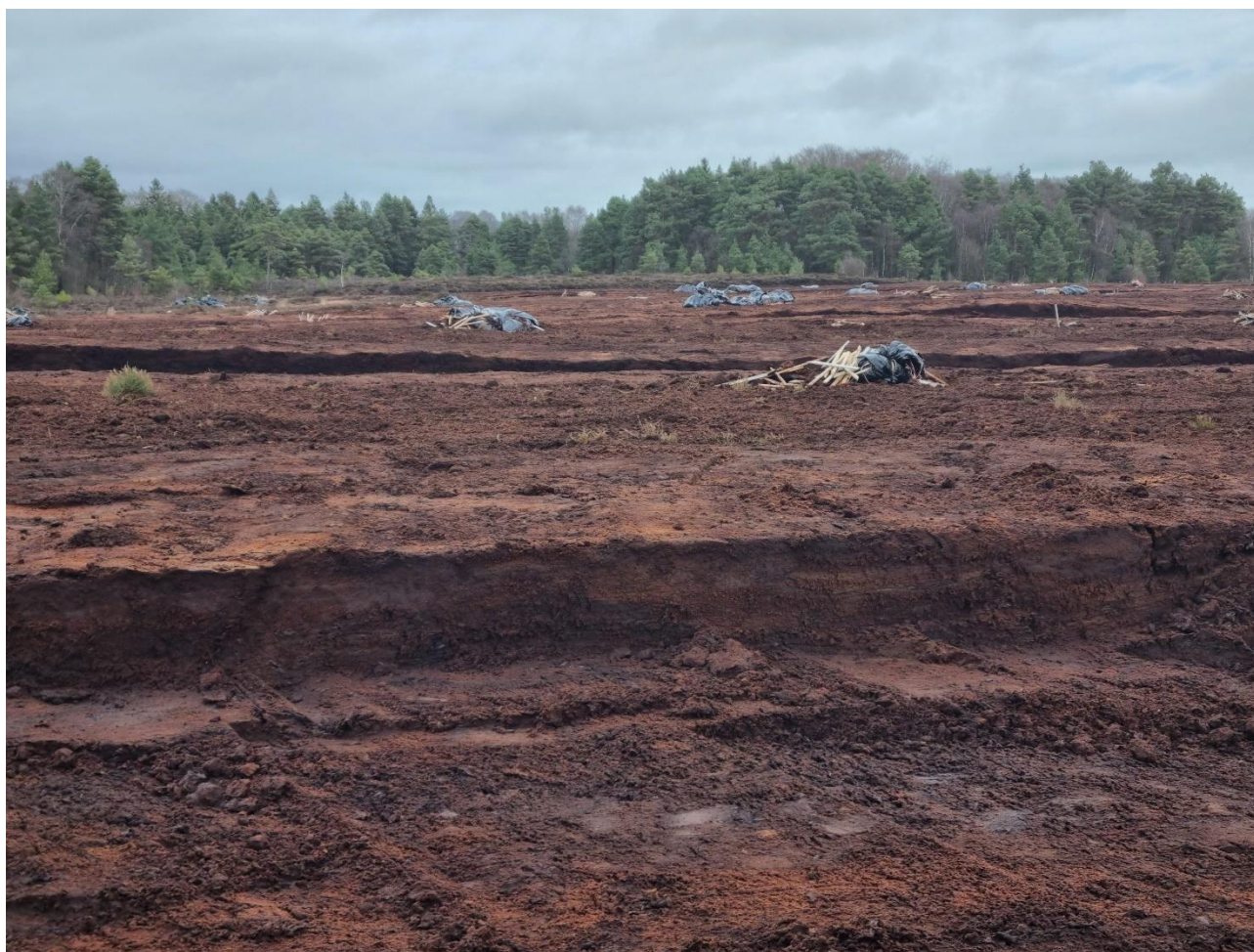
Photo 1: Photograph showing a section of the western/north western part of the peatland where clearing, drainage and preparatory works had recently taken place.
