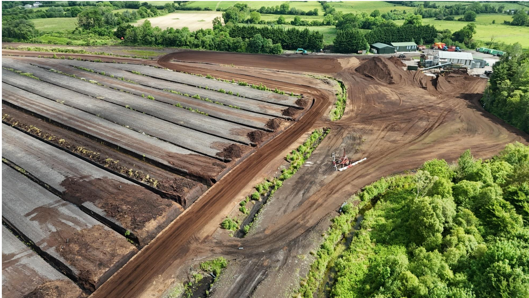
Photo 5: Drainage works noted on the peatland.
