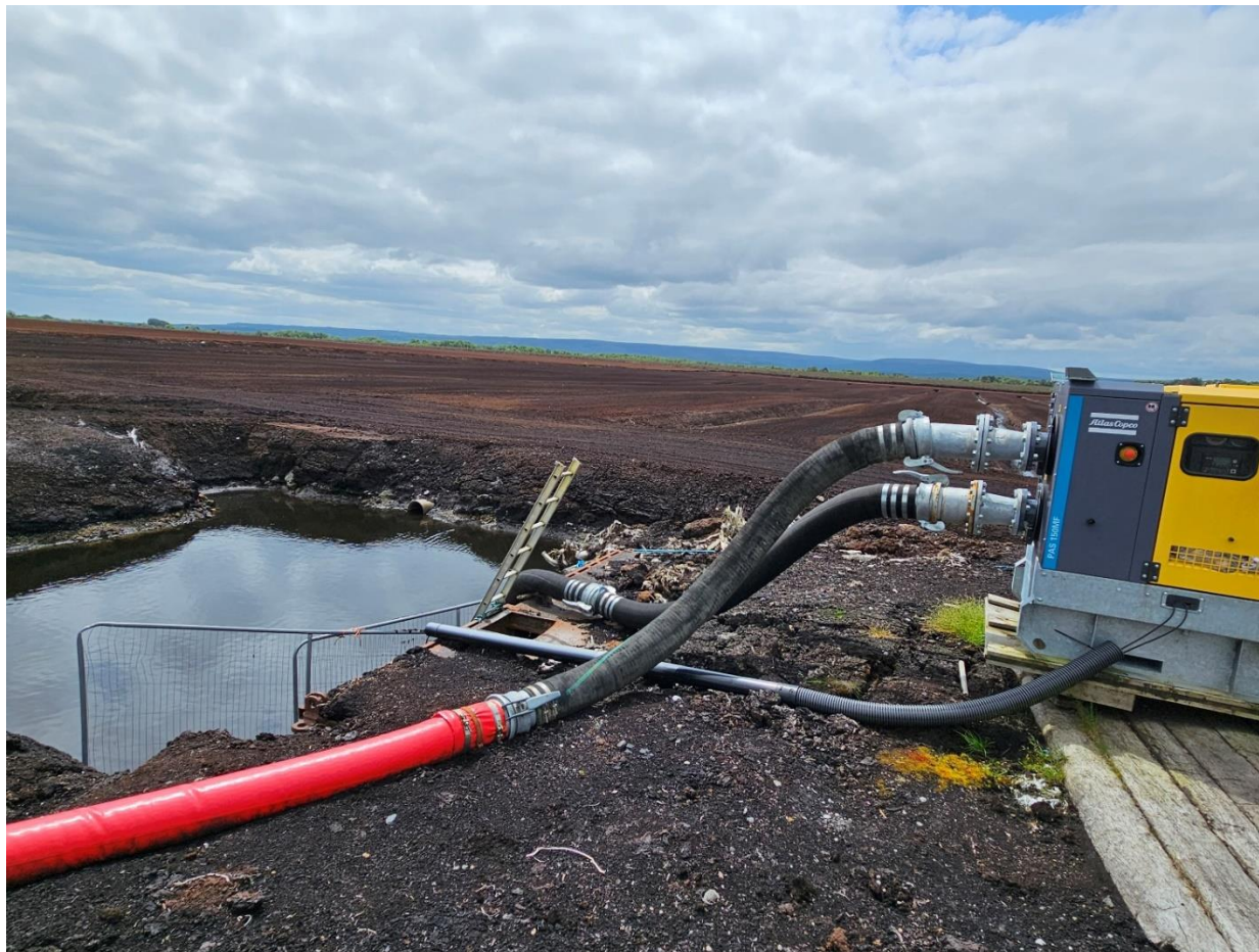
Photo 6: Water pump noted at one of sedimentation ponds.
