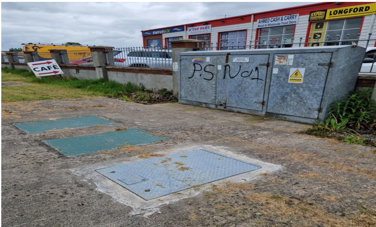
Figure 16 Pumping station at Mastertech / N63 with emergency overflow at bridge.
