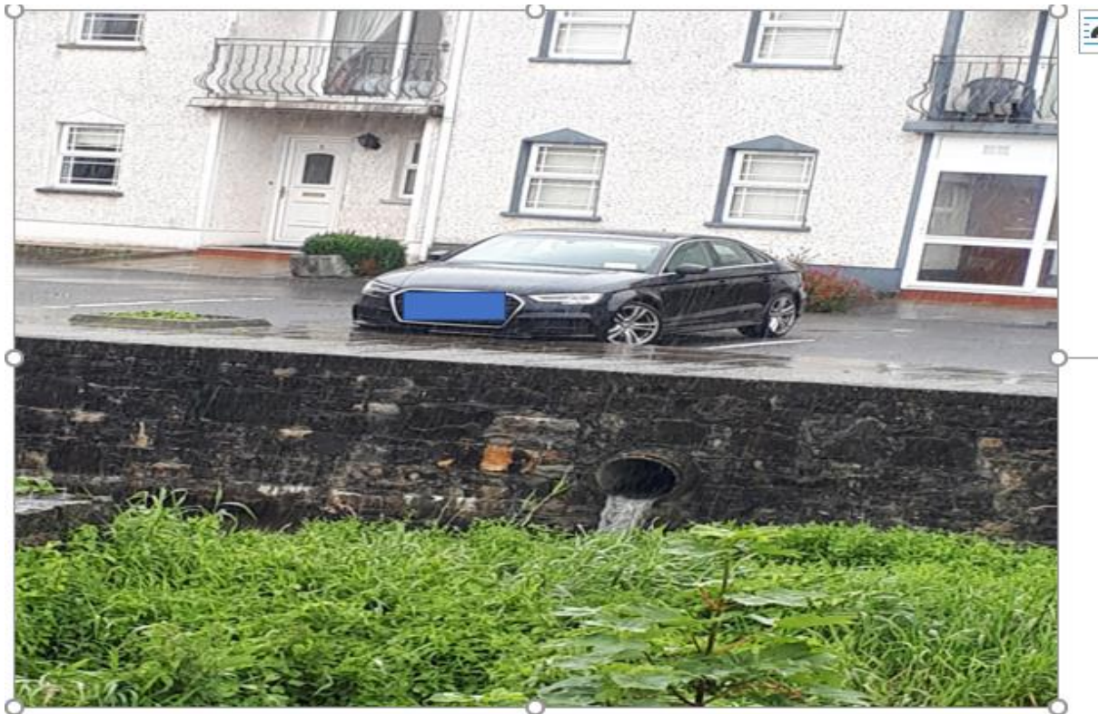
FIGURE 7 Contaminated Surface Water overflow at Church Street carpark.
