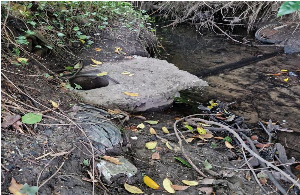
Figure 17 Overflow behind Ardnacassa Lawns estate
