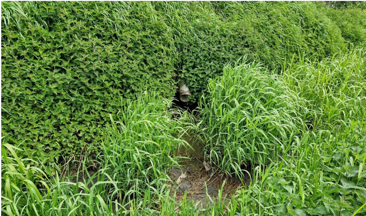
Figure 10 Surface water discharge pipes which may need further assessment at Connaught Road.
