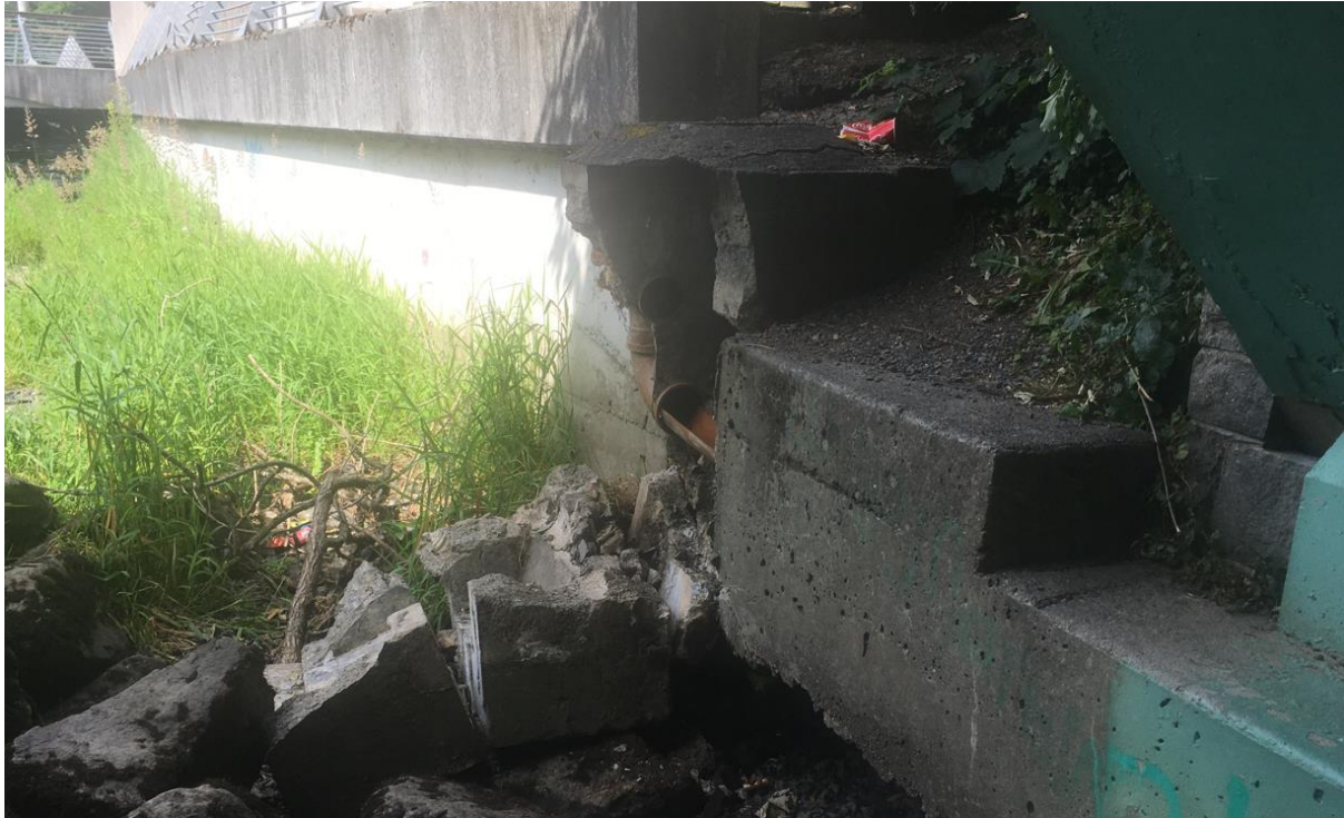
FIGURE 8 Collapsed sewer near the cinema which was rectified.
