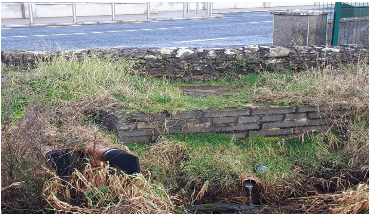
Figure 14 Discharge from a development led wastewater treatment at Stonepark that was referred to Longford County Council for further assessment.
