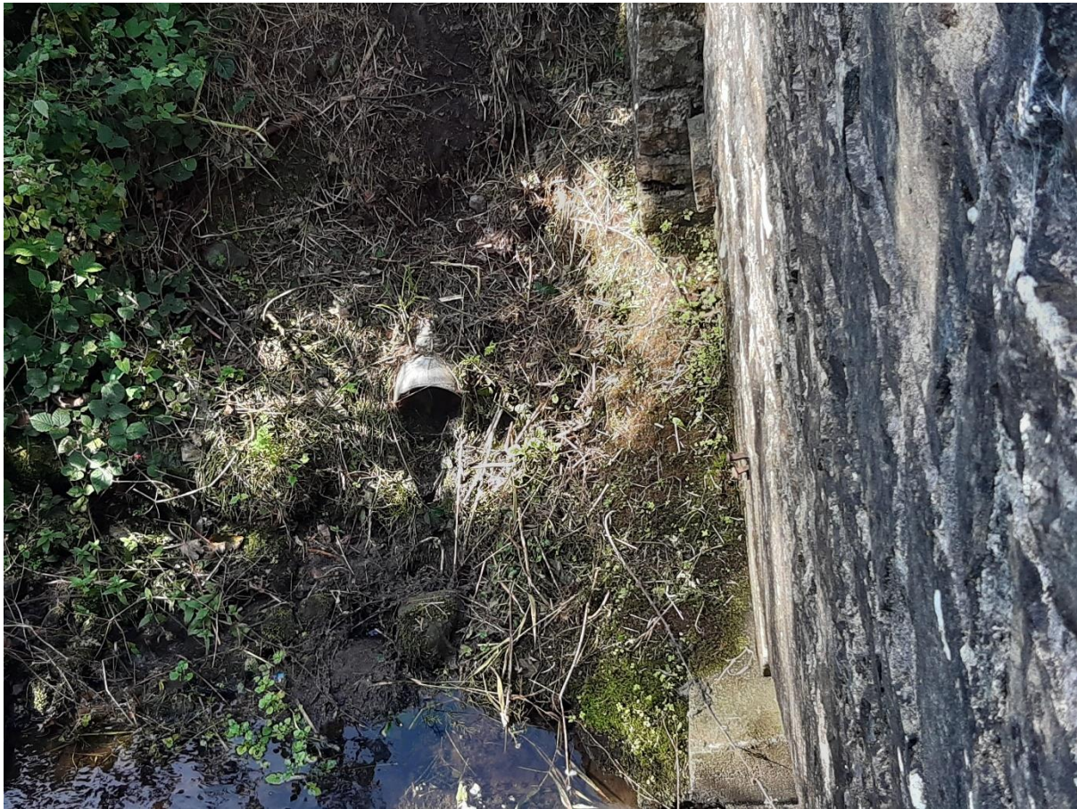
Photo C: Six-inch pipe protruding from the left bank, immediately upstream of the N5 road bridge as viewed from the bridge in September 2021 (LCA site 3.1.2, referred to as the misconnection discharge above).
