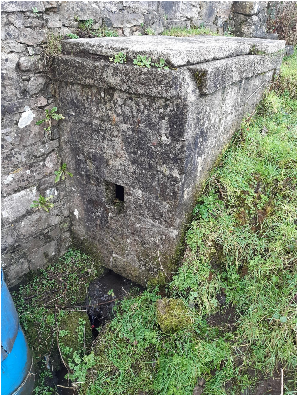
Photo B: Old stone/concrete tank at the base of the N5 road bridge from which water discharges to the Owennaforeesha River (LCA site 3.1.1).
