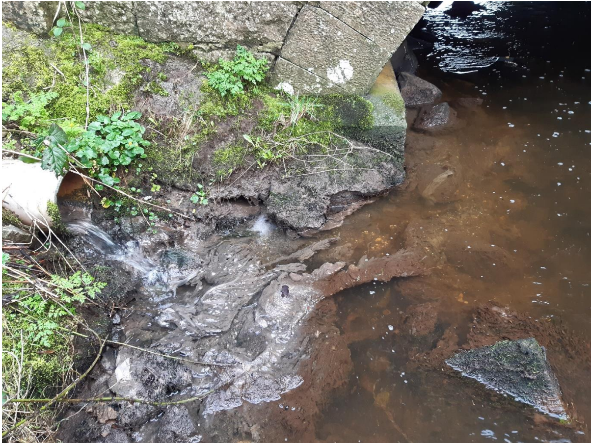
Figure 3: Raggings and sewage fungus below discharge from pipe at LCA site 3.1.2 on 15/2/2023
