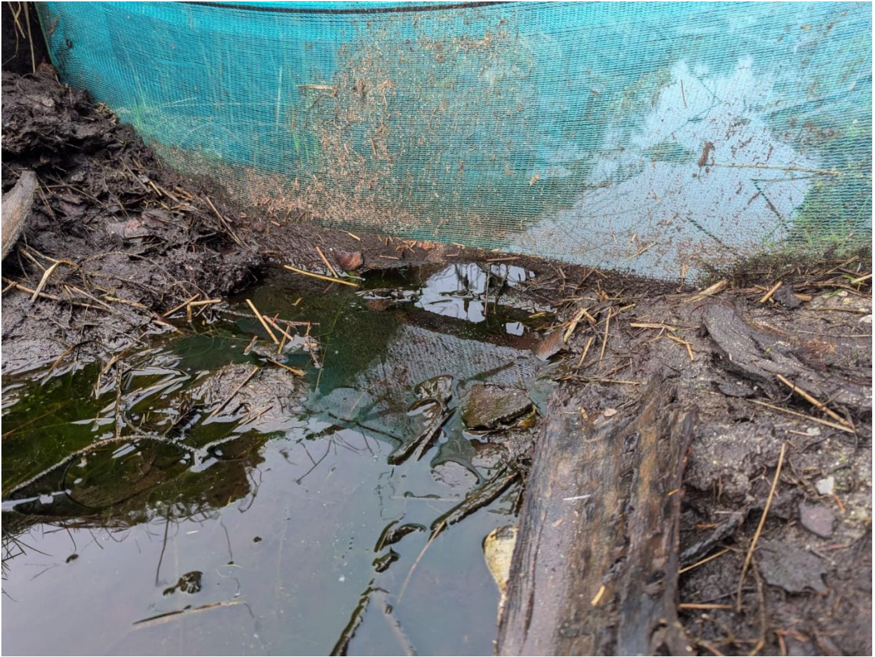
Image 15: Hole punched through sediment trap. Sediment visible beside trap.
