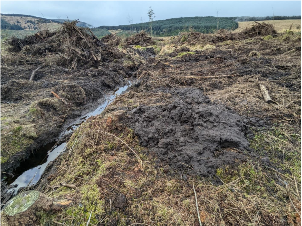
Image 2: Significant peat disturbance at RWC crossing point.
