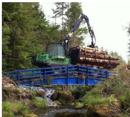
Figure 17. Mobile prefabricated bridge used as a temporary crossing over sensitive aquatic zone.
