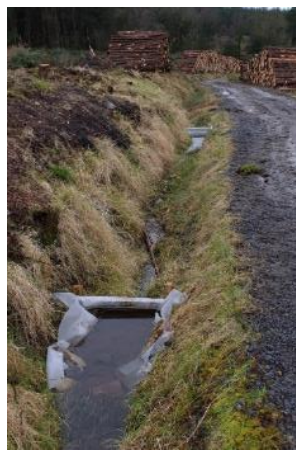
Figure 19. Silt traps placed in series in a roadside drain
